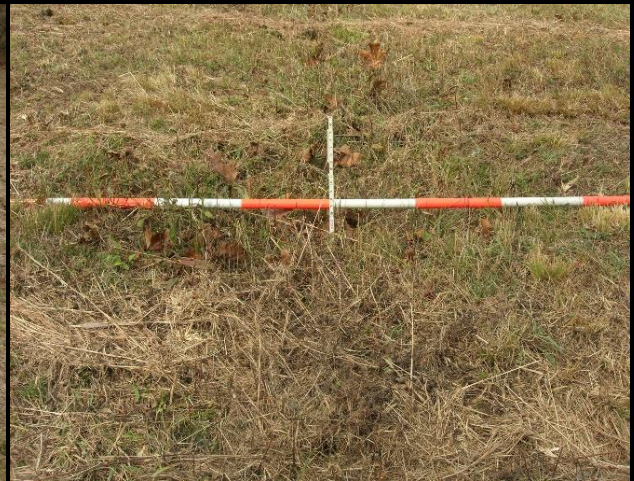
Image 10: Depression in downstream slope near toe, looking upstream
