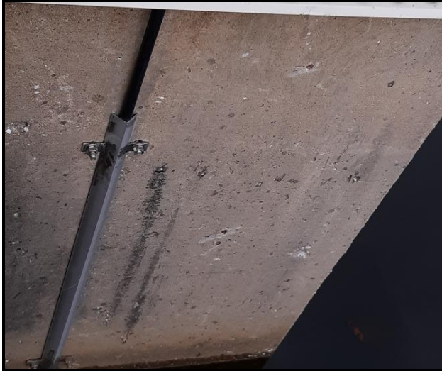
Image 43: Water intake tower minor concrete damage
