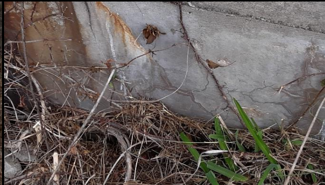
Image 48: Cracks and efflorescence at base of right side of stairway
