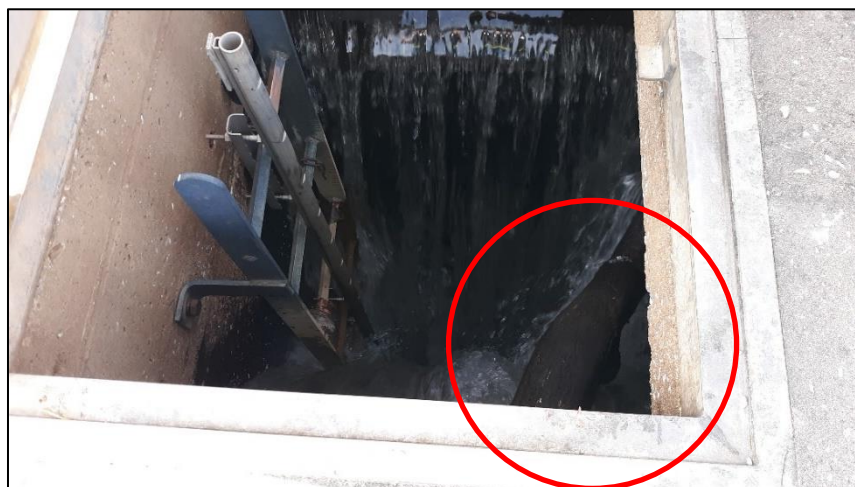
Photograph 6: Log lodged in principal spillway riser.
