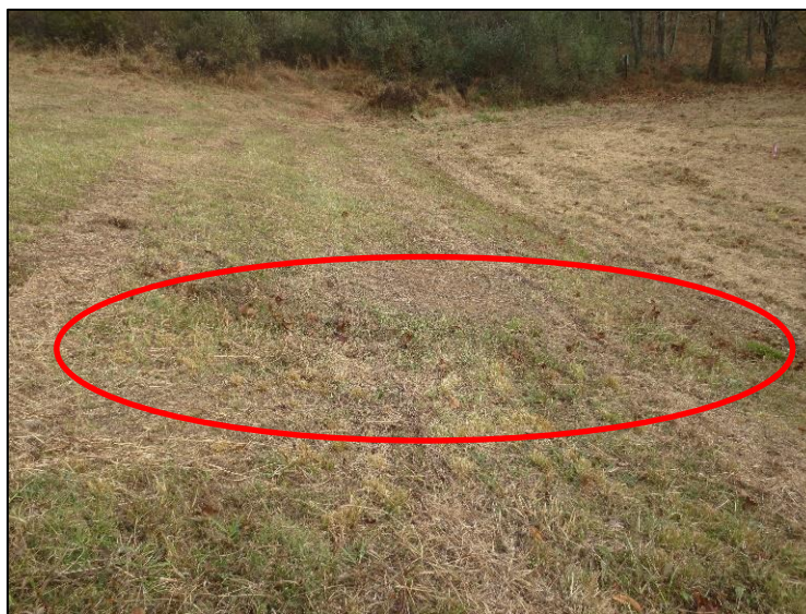
Photograph 3: Downstream embankment slope depression.
