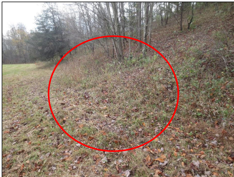
Photograph 8: Colluvial pile on outside auxiliary spillway slope.
