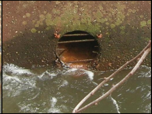
Image 26: Damaged left toe drain animal guard
