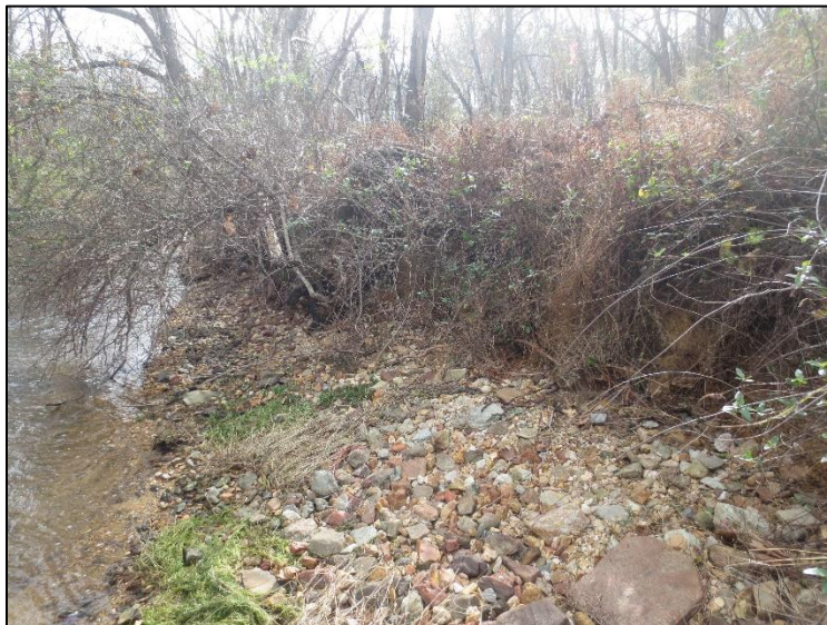
Photograph 7: Erosion and undermining on right outlet channel slope.
