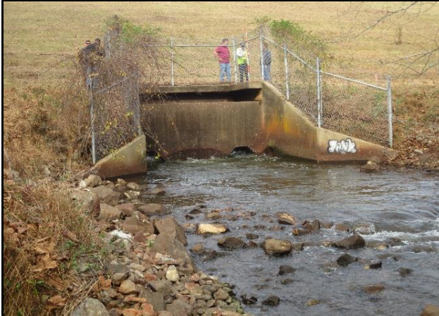
Image 21: PSW outlet impact basin
