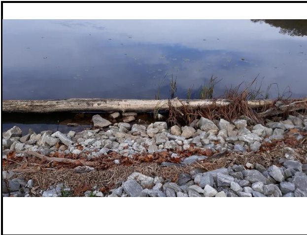
Image 7: Debris and small riprap at upstream waterline
