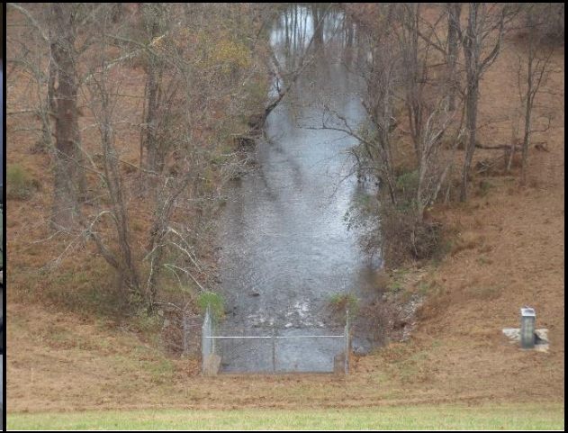
Image 20: PSW outlet channel
