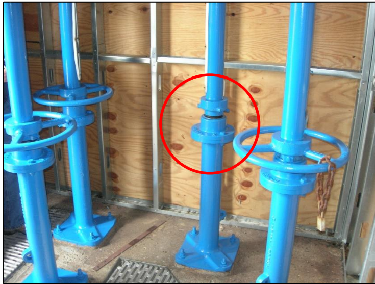
Photograph 10: Handle broken off the hand operator handle.
