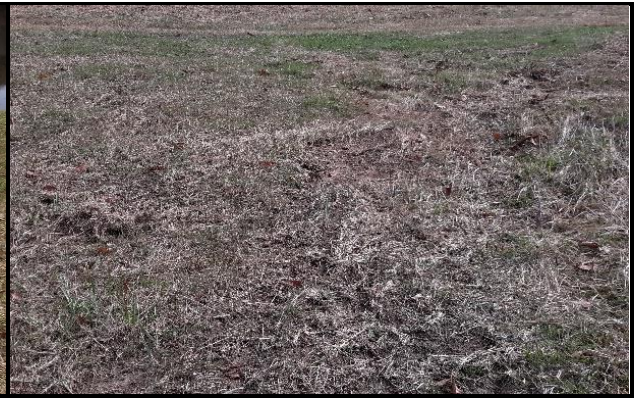
Image 14: Bare spots on left upstream abutment
