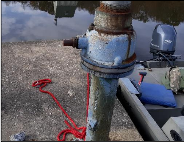
Image 19: Lake drain gate wheel
