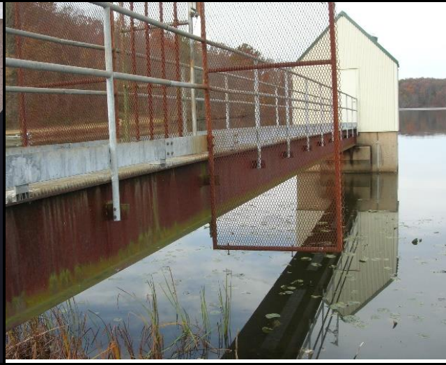
Image 44: Catwalk support beams; rusted gate
