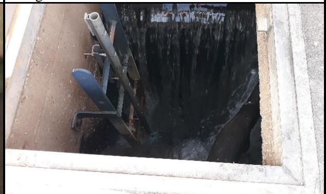
Image 18: Inside of PSW riser. Note log lodged in inlet
