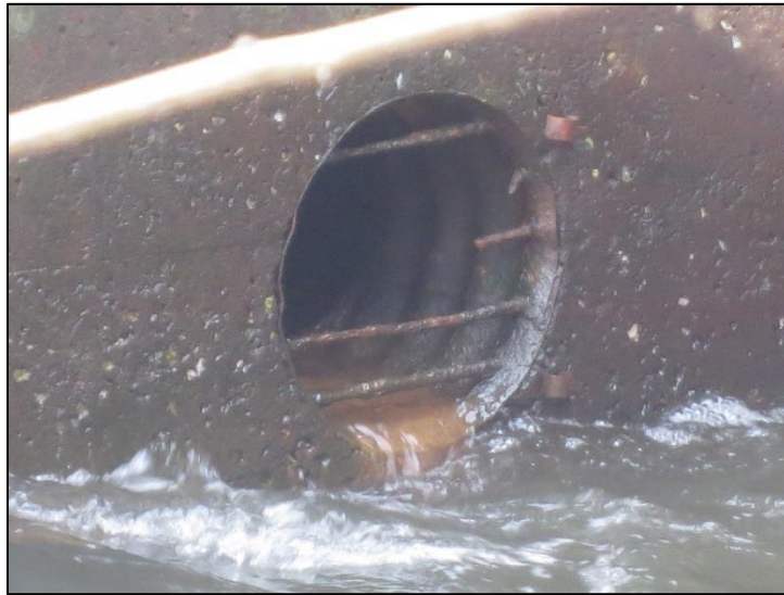
Photograph 5: Damage to right drain animal guard.
