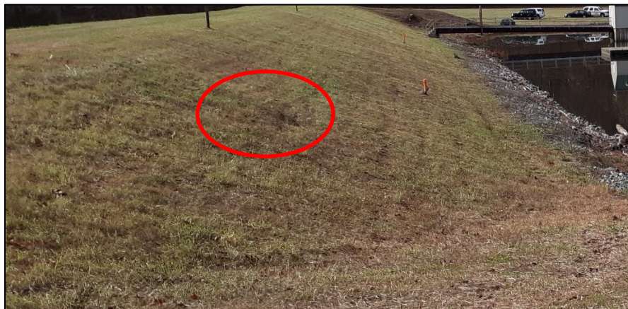
Photograph 2: Upstream embankment slope depression.
