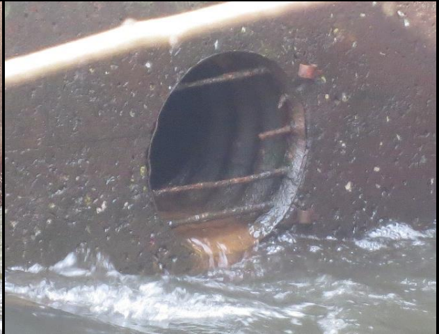
Image 24: Damaged right toe drain animal guard
