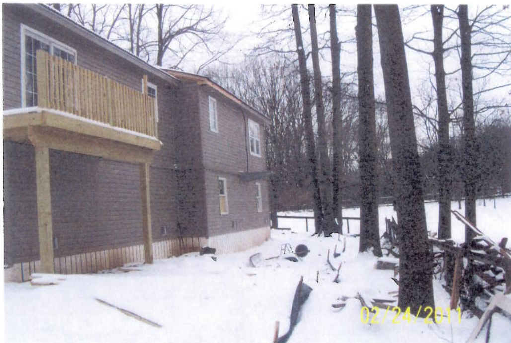
REAR VIEW(w/ HVAC Cantilevered Pad) - 2/24/11
