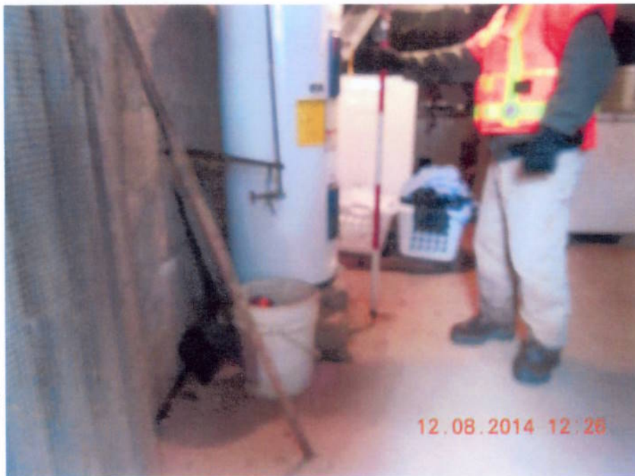
Lowest Machinery View 12/8/14
