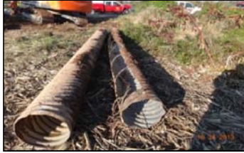
Photograph of deteriorated metal pipe
