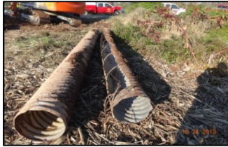
Photograph of a deteriorated metal pipe.
