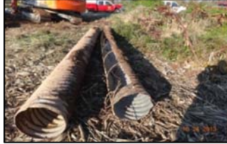
Photograph of a deteriorated metal pipe.
