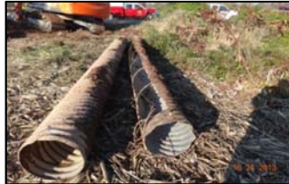
Photograph of a deteriorated metal pipe.
