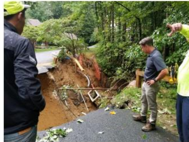
A flash flood in northern Harford County caused major damage to approximately 20 roads and culverts, as streams rose 11 feet above normal water levels on August 31, 2018.
