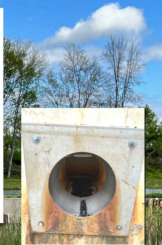
Orifice w/ U20L H0BO Pressure Sensor Installed 2022
