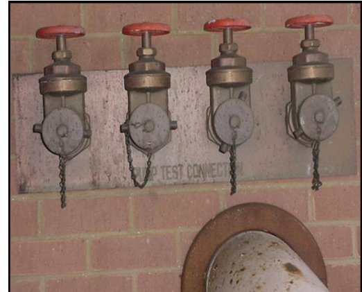
Fire Pump Test Header
