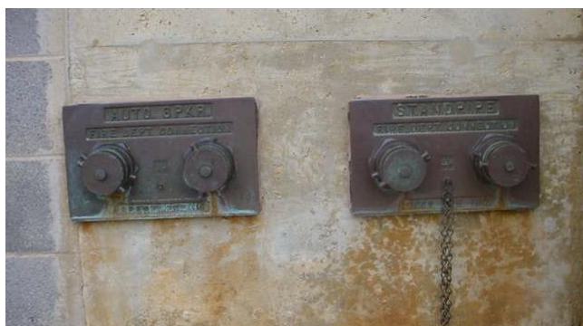
Adjacent, but Separate Sprinkler and Standpipe Connections
